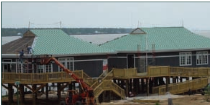
New buildings in final phase of construction with dedication planned on June 19, 2008
